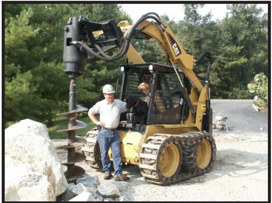
Rusty Wayne takes a break with his dogs at a job site in Ohio. He uses the Eskridge S7848 auger drive on a CAT 248 skid steer to drill holes for building foundations.
